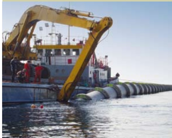
Outfall pipeline DN/ID 1800 mm
